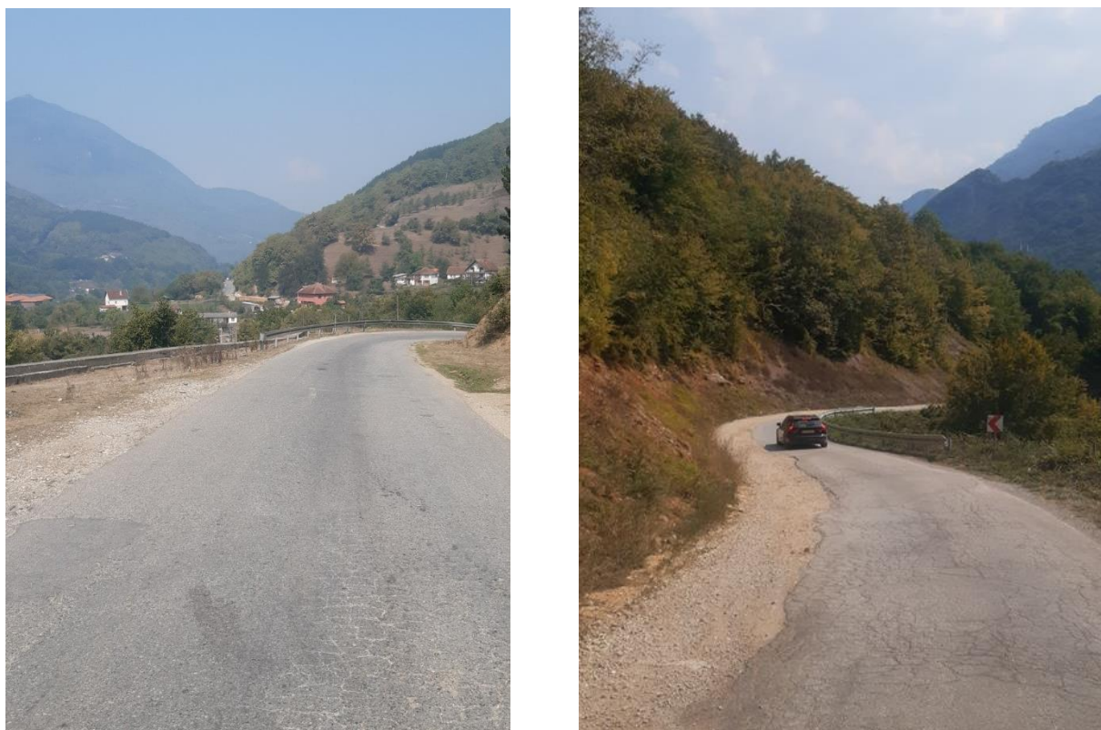
Figure 2: Current state of the M-18 road: section B
