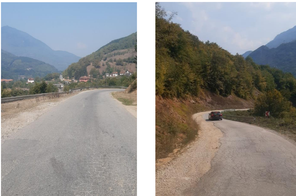
Figure 2: Current state of the M-18 road: setion B
