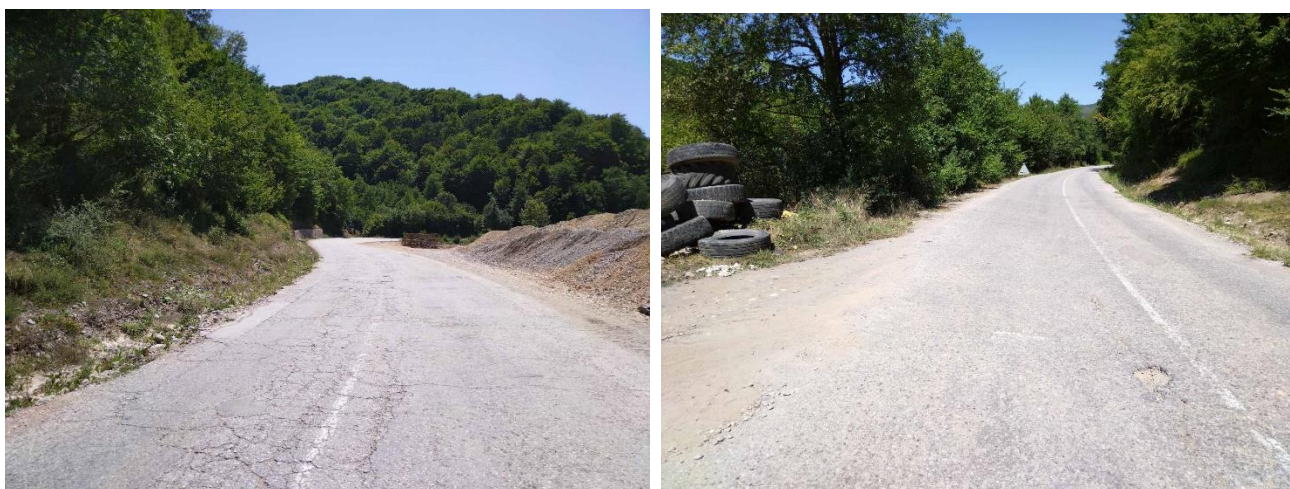
Figure 1: Current state of the M-18 road: section A
